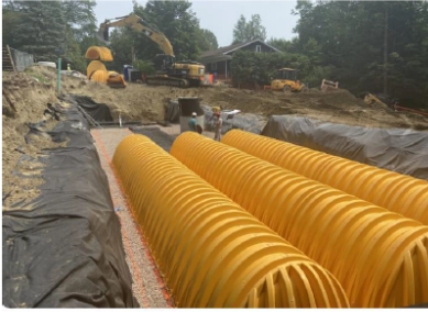
Dry Wells and Detention Chambers
